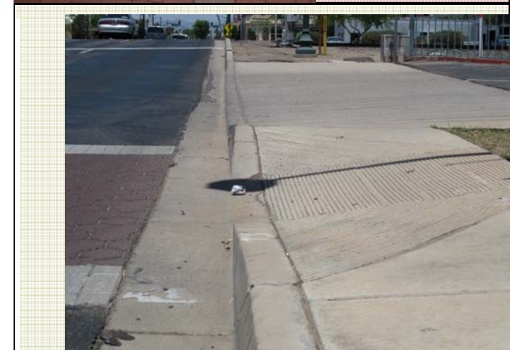
Unfavorable: Sidewalk patterns interrupted by driveways and ramps having steep cross slope
