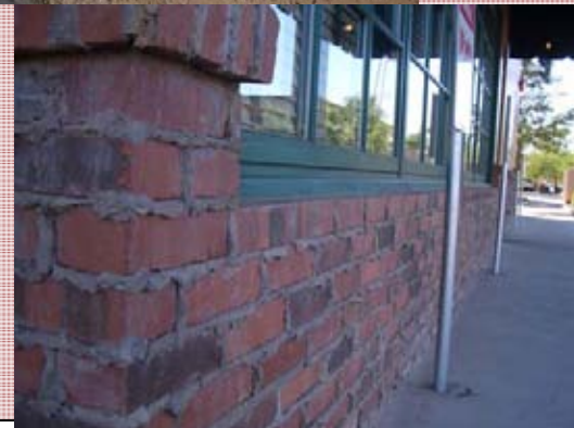
Favorable: Aged Brick anchoring building base
